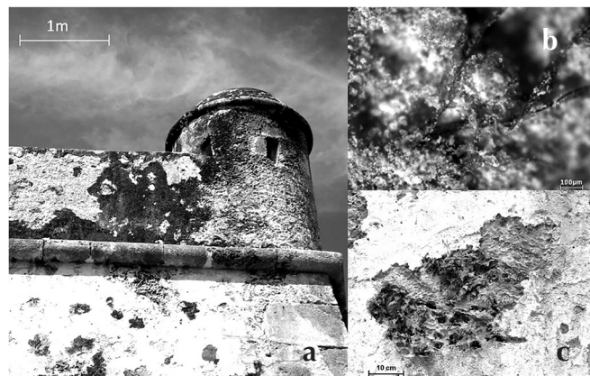
FIGURE 4. Biological activity at the San Carlos Bastion: (a) General view of biological colonization formed over east wall; (b) Mortar disintegration induced by hyphae penetration; (c) Mortar damage —consequence of biological activity— (Photograph: Javier Reyes, 2010).
