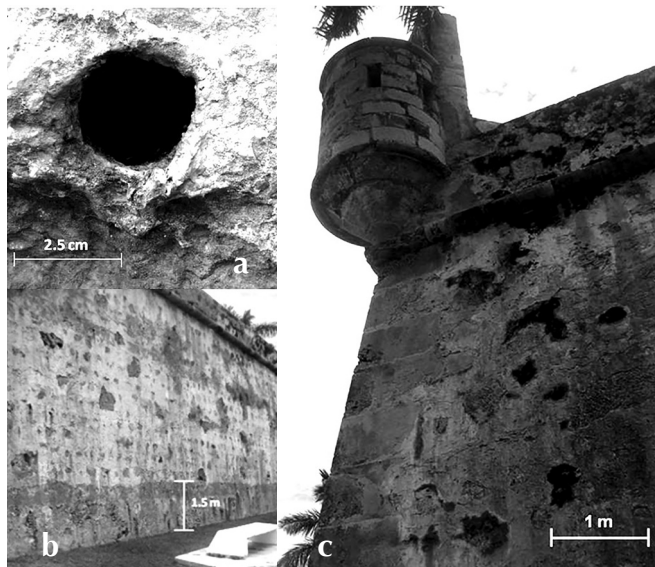
FIGURE 2. Different weathering effects at San Carlos Bastion: (a) Water discharge structures. Efflorescence and crust formation can be observed outside; (b) Alternation stripe observed at the north wall; (c) Preferential limestone quarry block degradation at west wall (Photograph: Javier Reyes, 2010).
